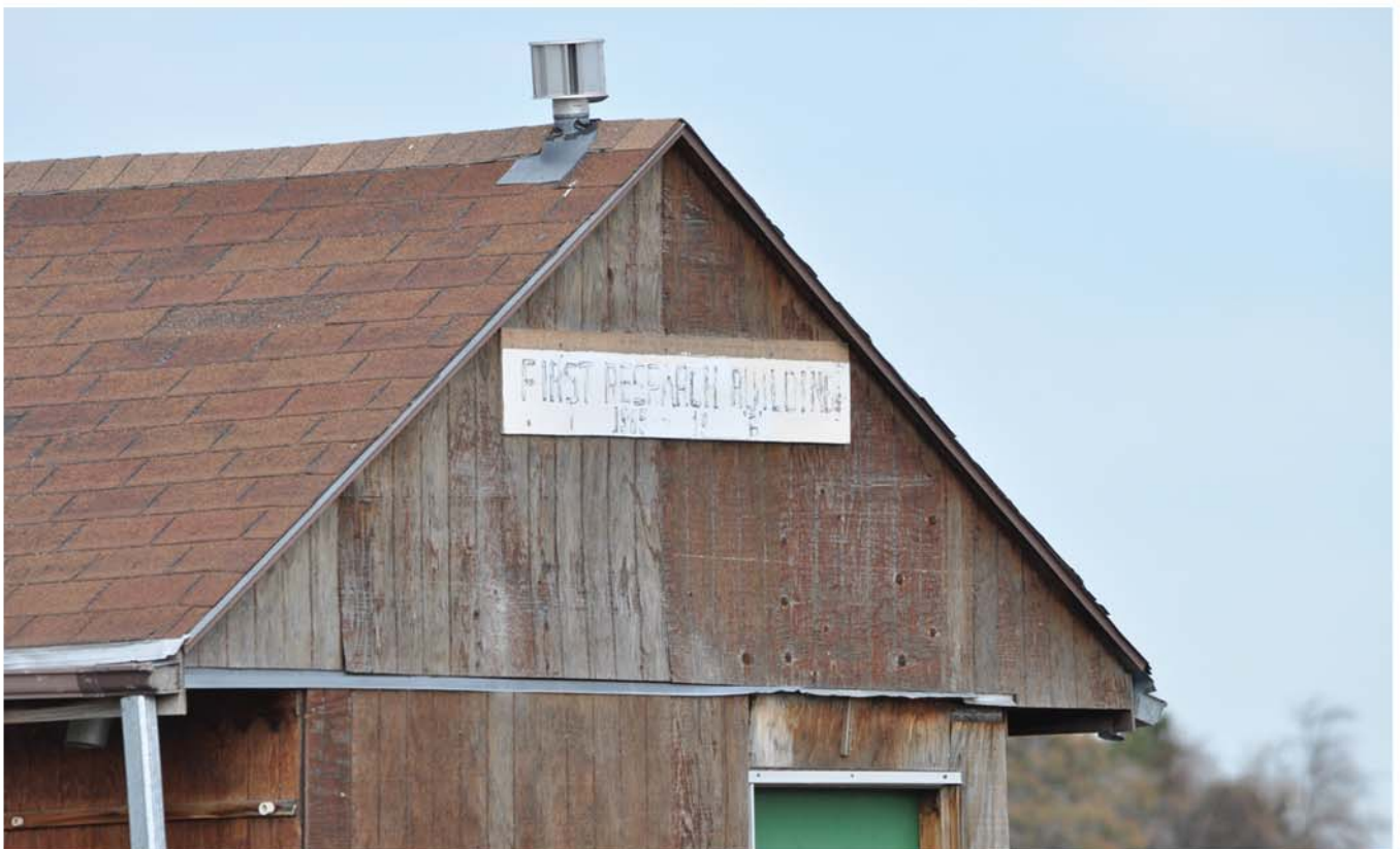
5AH3453_2: Close-up view of sign located on east wall gable above the door. The sign reads, "First Research Building 1985-19_B"
