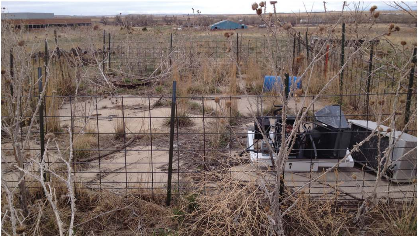
5AH3451_1: View southwest showing area of concrete slab at north end of building foundation
